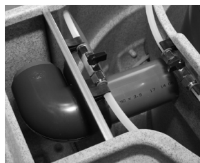
Figure 17.3 - By-pass in operation
